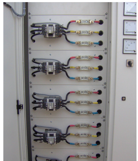
Contactors and HRC Fuses
