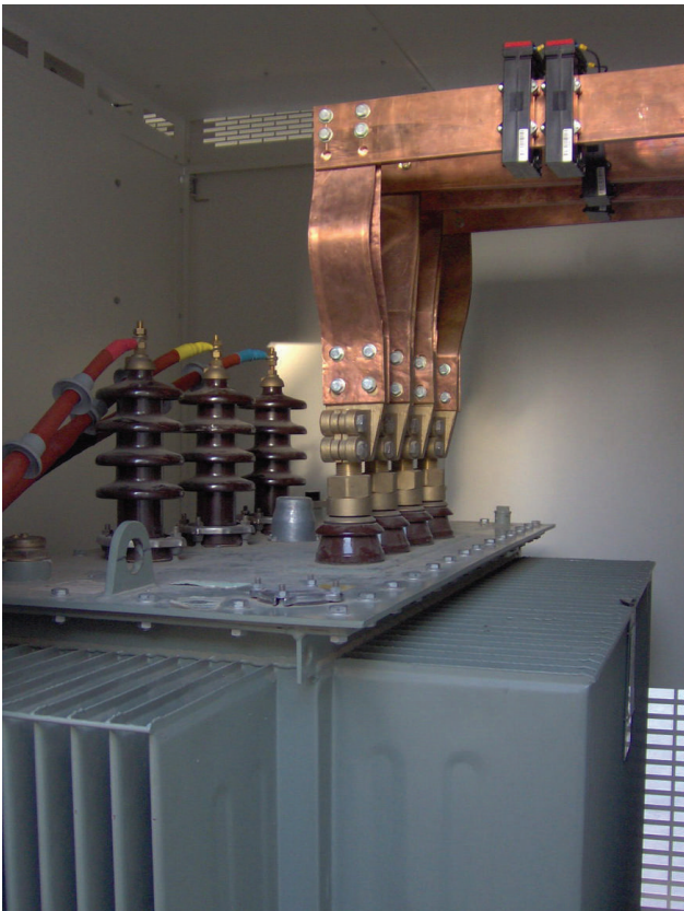
Transformer inside the Kiosk
