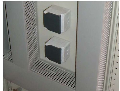
Duct & Power Socket
